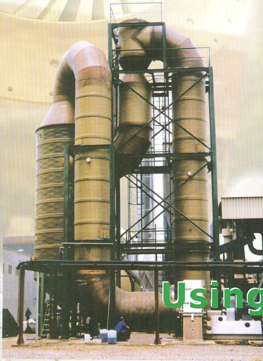
Dedusting unit (venturi-cyclon) on a liquid manure treatment plant 某液体化肥厂的除尘单元（文丘里+旋风分离器）
