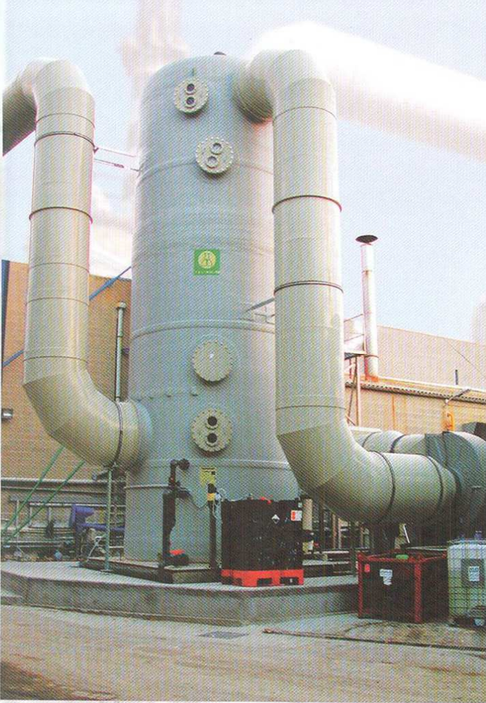
NOx chemical absorption at an Asian chemical industry 亚洲某化工厂的NOx化学吸收装置
