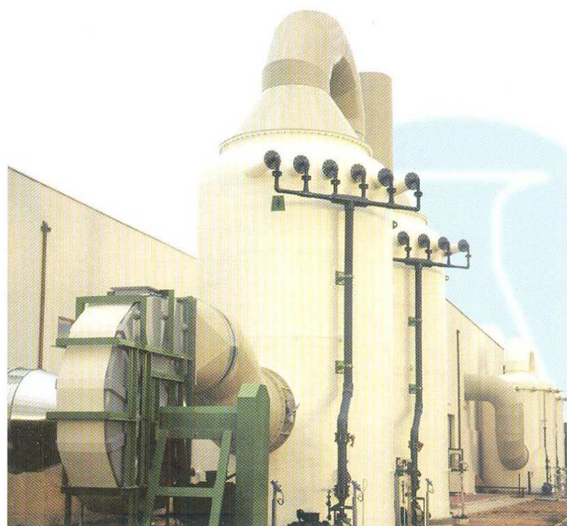
NH 3 +H 2 S+R-SH absorption on an industrial WWTP 工业废水处理厂的NH 3 +H 2 S+R-SH吸收装置
