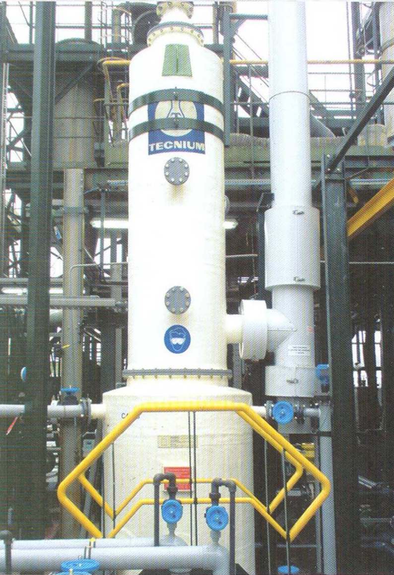
VOC absorption on a pharmaceutical plant in France 法国某制药厂的VOC吸收装置
