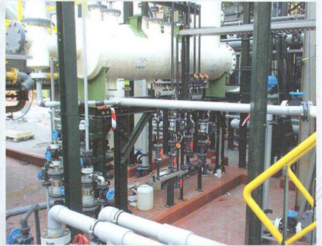
Dedusting unit by multi-venturi on a pigment manufacturing plant 某染料厂的复合文丘里除尘系统
